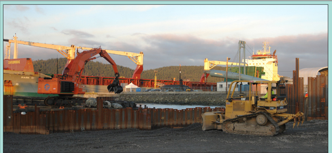
COMMUNITY TOUR: Work continues at Dakota Creek Industries (DCI) on a joint Port/DCI project called "Project Pier 1." Another community tour of the project is scheduled Monday, January 12. Call 293-3134 to RSVP for the 4 p.m. tour.
