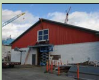
Crewmen wrap up work on the west side of historic Port Warehouse 4 at the end of Commercial Avenue.
