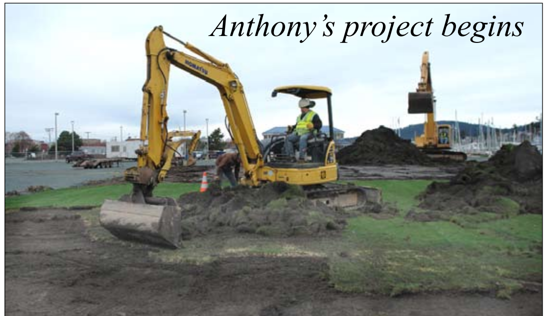
Monday, March 1 marked the start of site preparation for an Anthony's restaurant to be located on the shoreline at Cap Sante Boat Haven. The seafood restaurant will be located near the esplanade overlooking the marina, just north of the boat launch and the commercial fishing dock.
