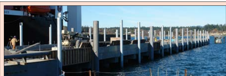
DCI CONTINUES PIER WORK: Project Pier 1, a cooperative partnership between the Port of Anacortes and Dakota Creek Industries (DCI), dates back several years. Among shipyard improvements is this pier extending into the Guemes Channel. The pier will make it possible for the shipyard to bid additional projects.
