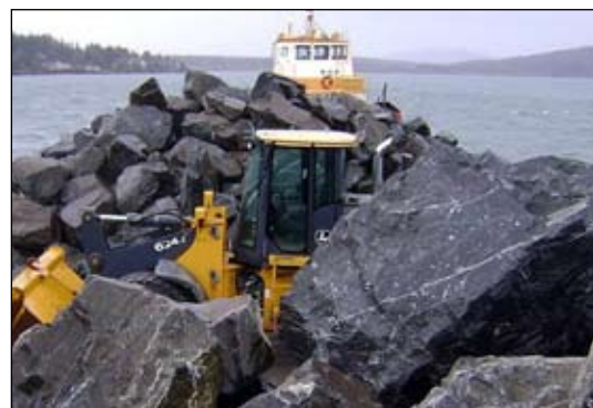
This photo of heavy equipment and rock for new breakwater illustrates the size of raw materials.
